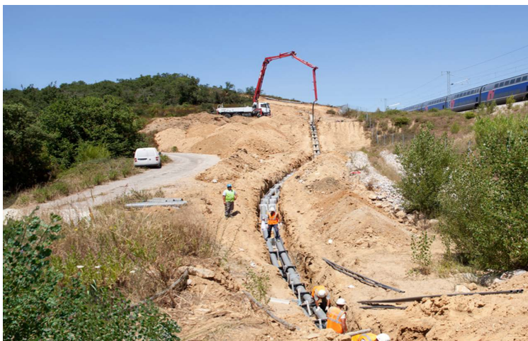
Figure 2.2 View of an undergrounding section of the RTE / RED INELFE HVDC \pm 320 kV Interconnector France-Spain project.
