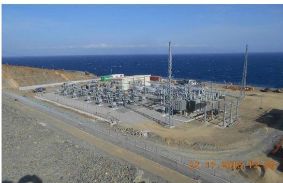
Figure 1.4 The SVC substation on Syros island
